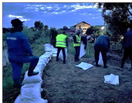
Fig. 7b Jiu Water Basin Administration intervention by raising sandbag piers in Cernătești settlement (Source: Cuvântul Libertății, 06.06.2023)
