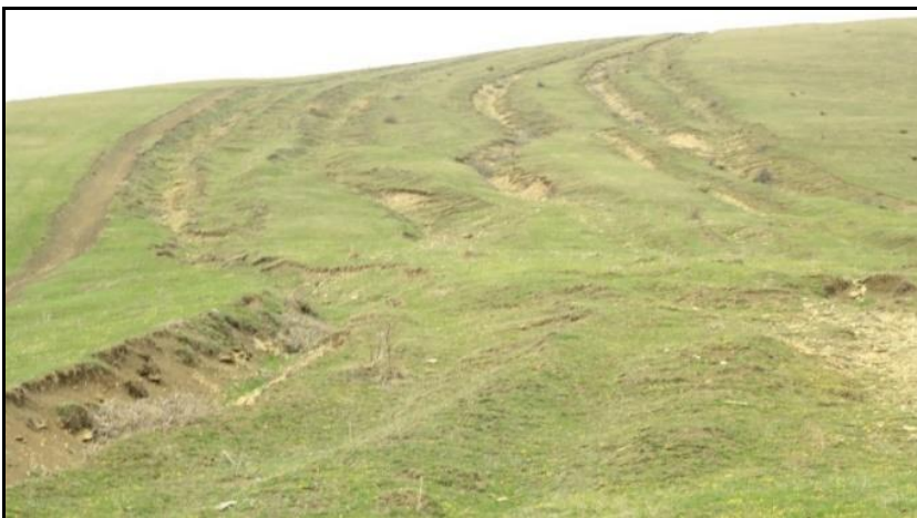
Fig. 5. Gullies, developed on a slope affected by landslides
