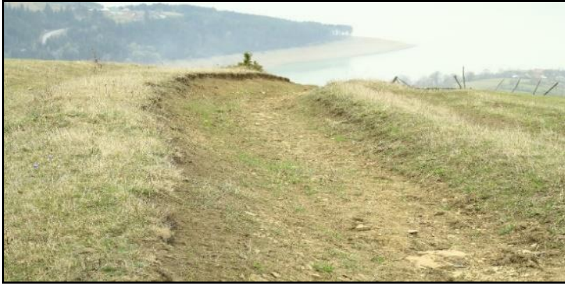
Fig 3. Road affected by erosion in Tulghes
