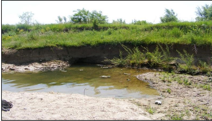
Photo no. 8. Slope collapse (subsidence) - Guești
