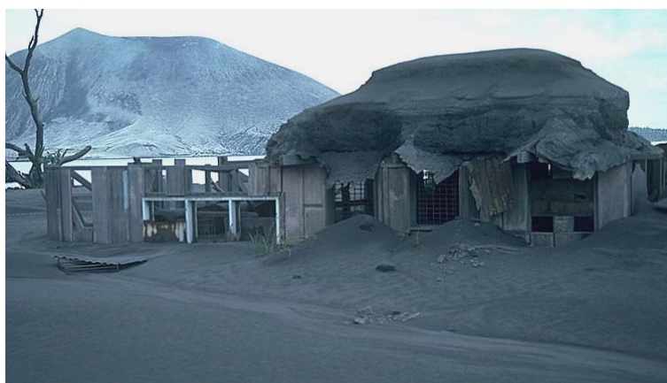
Fig. no 2. House damaged by the heavy load of ash that accumulated on its roof during the eruption of Rabaul Caldera in Papua New Guinea on September 19, 1994. Note the thickness of ash deposits on top of the roof that did not collapse (right side). For a layer of ash about 10 cm thick, the extra load on a building can range 100-125 kg/m 2 . One of two volcanoes that erupted is visible to the left of the house. Photo Credit: E. Endo, October 1994.
